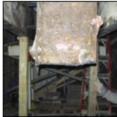
This photograph shows the clipped pier. With temporary bracing in place, the stone cladding, brick fill and steel column section can be removed safely.
