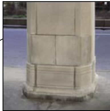
Removal of the stone cladding at the base of the pier revealed slight deterioration of the steel support. This picture shows the area of the investigative opening. Once the repairs were completed, the stone was restored to its original condition.
