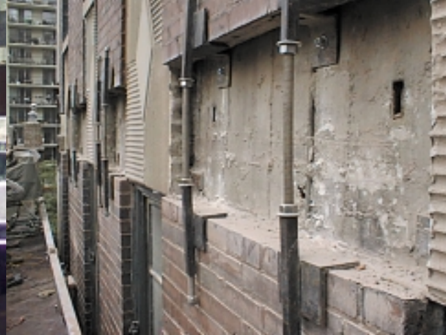
Below: Bracing support system at 73 East Elm Street.
